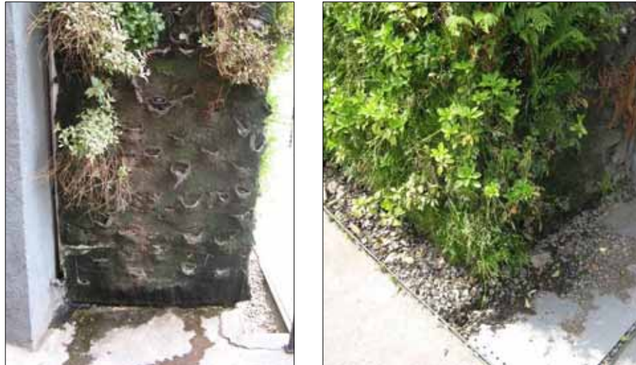
Figure 3.22 Left photograph Caixa forum in Madrid; bare surface of the vertical placed panel, water leakage and degradation of the substrate is visible (felt pockets). Right photograph belongs to the same façade were they solve the leakage with a gutter filled with gravel for drainage and avoiding splashing of water droplets (Photos Barbera Peters).
