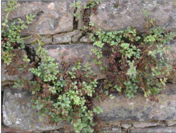
Figure 3.4a Characteristic wall vegetation typically on older constructions created with limestone mortar joints.
