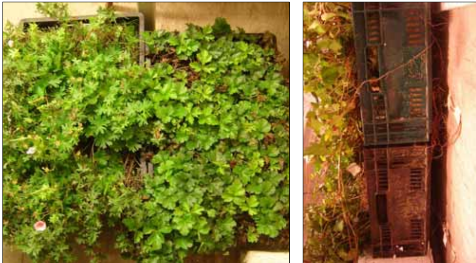
Figure 5.72 A living wall system based on foam substrate, thickness of the foam is 18 cm. Again an air cavity is visible of 5 cm between panel and façade. Plant species used for this test are Geraniums.
