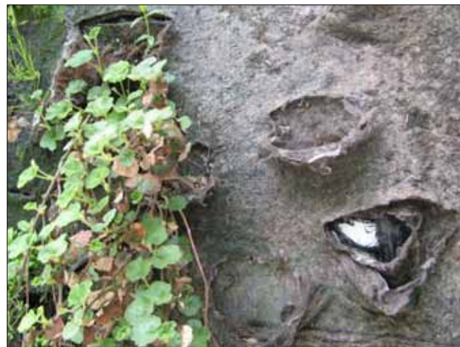
Figure 3.23b Maintenance in the case of a living wall system (based on felt layers) includes: checking the integrity of the substrate(s), functioning of the watering system and replanting of bare parts of the façade.
