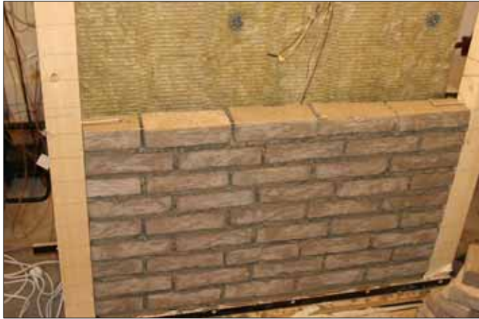
Figure 5.21 Finishing the outer masonry it is also possible to see the wires for thermocouples and humidity sensors as placed inside the bare wall.
