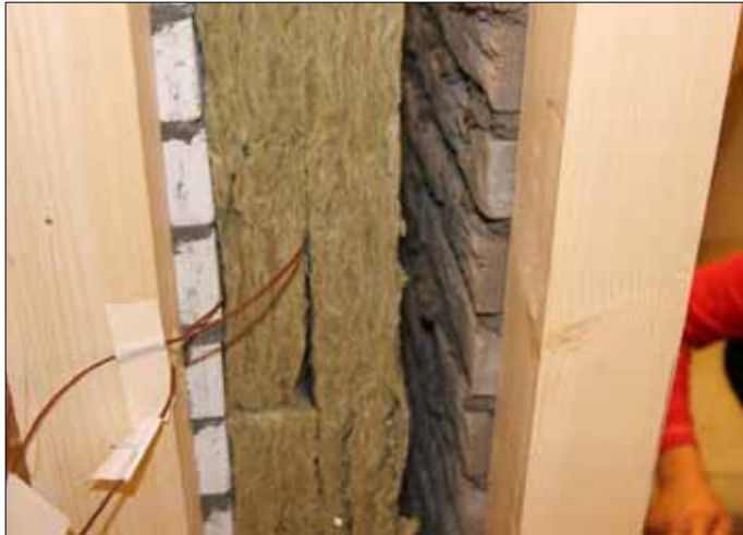
Figure 5.22 Cross section of the different layers of the bare wall; from left to right: limestone, mineral wool, air cavity and the masonry of clay.
