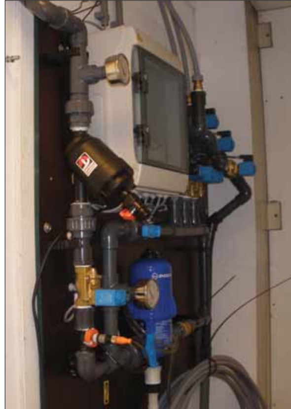
Figure 2.20: self-automated watering and nutrition system for living wall systems at Ford building in Amsterdam (source: Middellie, 2009).
