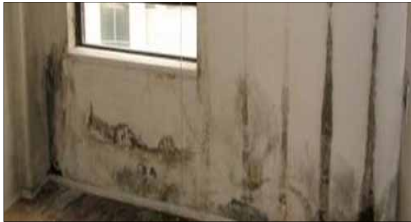
Figure 5.3: damage inside the building because of humid walls (source: www.devochtbestrijder.nl ).
