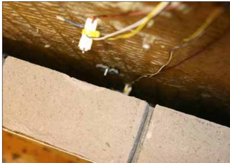
Figure A.4: humidity sensors inside the air cavity, photo made during the construction.
