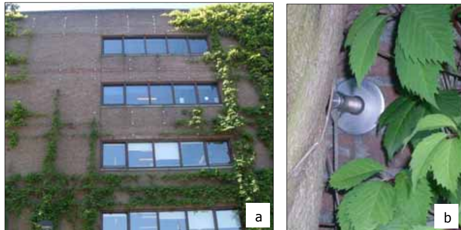
Figure 2.9: (a) and (b) cable and wire-rope net system (building EGM architecten, Dordrecht).
