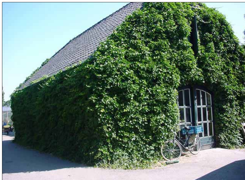
Figure 5.4: evergreen plants protect the building against the rain in all seasons (source: www.tomgarden.nl ).
