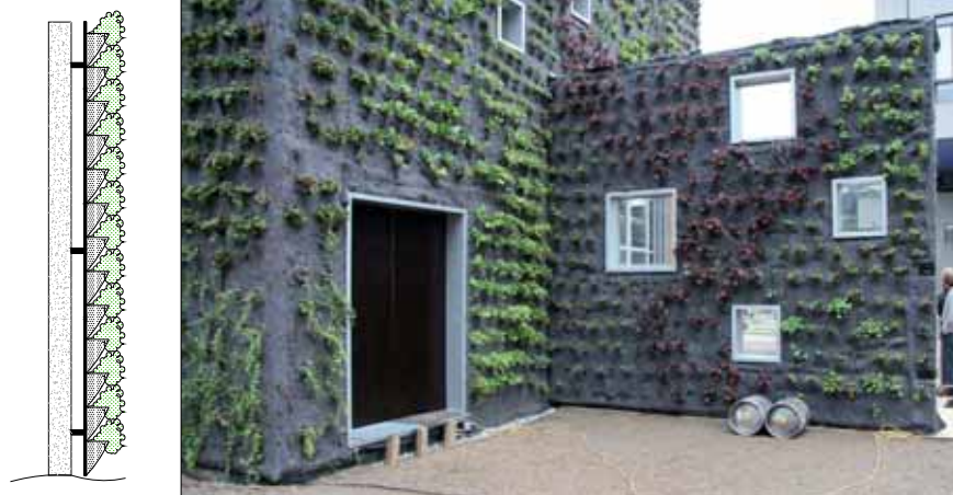
Figure 2.33: left, the principle of felt layers system; right, felt layers system in practice ("Black box", Stylos pavilion, Faculty of architecture TUDelft) (source: Geus, 2007).
